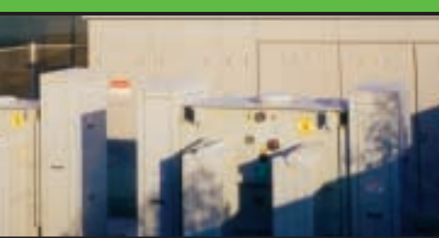
New 16.5 KV switchgear and transformers installed by AJK&A's Sam Sandoval and crew
