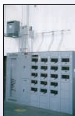
One of 10 power centers designed furnished and installed by AJK&A.
