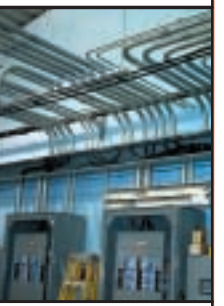
Electrical Switchover at KCSI-TV
