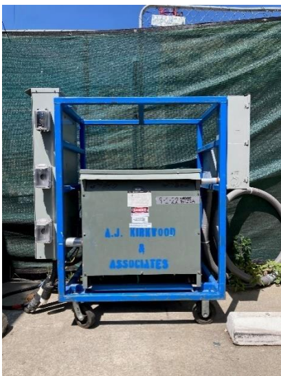
← Spider Boxes and Temporary Transformers: Duct tape, date, initial, mark "Tested OK".
